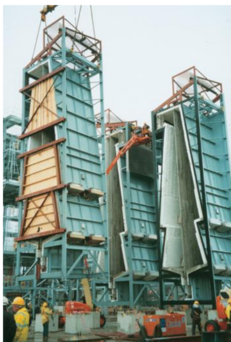
Figure 7 – Wood’s Terrace Wall Reformer [6]
